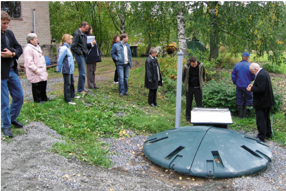
Figure 8. An example of a commercial package-plant as installed. Photo Satu Miettinen.
