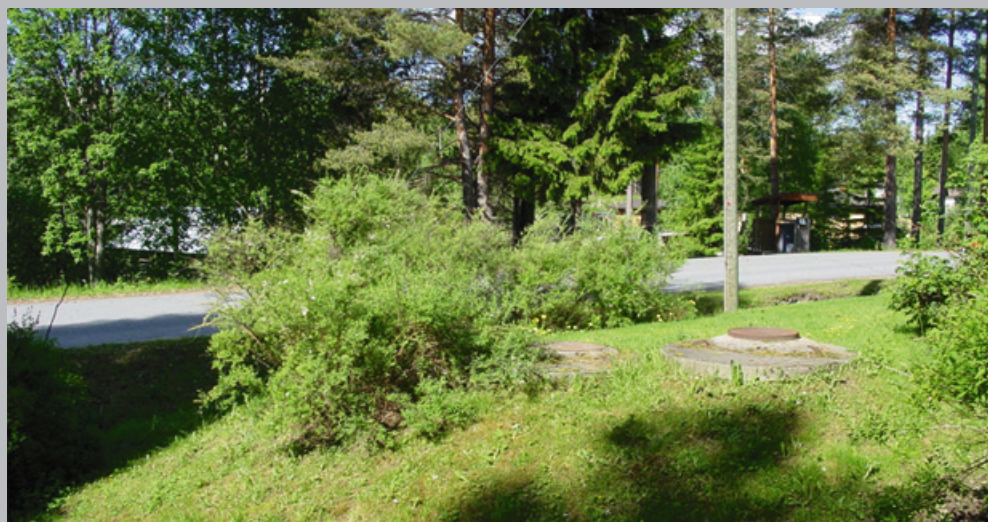
Figure 12. Two septic tanks and a leach field in a small building site which will have to be replaced by a new treatment system. Photo Eila Kaartinen.
